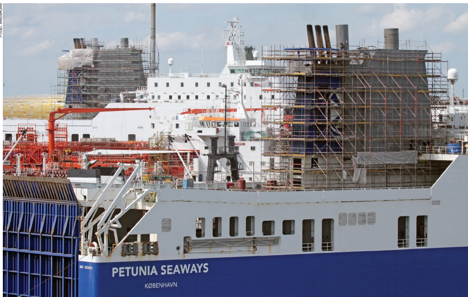
Petunia Seaways during scrubbers installation. In the background another DFDS Seaways ship while the similar operation was being performed.
